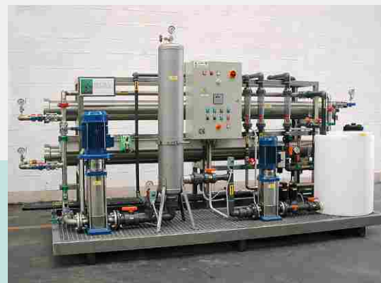
Reverse Osmosis unit - 7 mc/h
