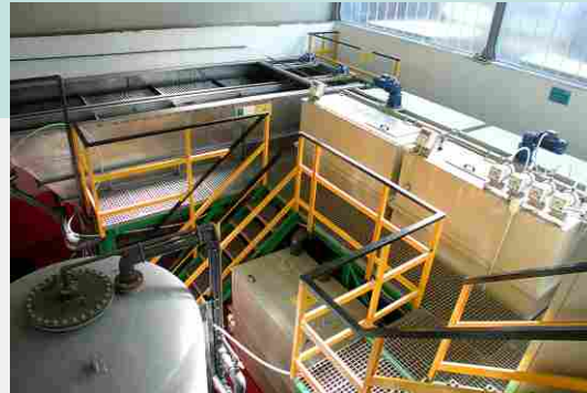
Chemical-physical plant - 30 mc/h
