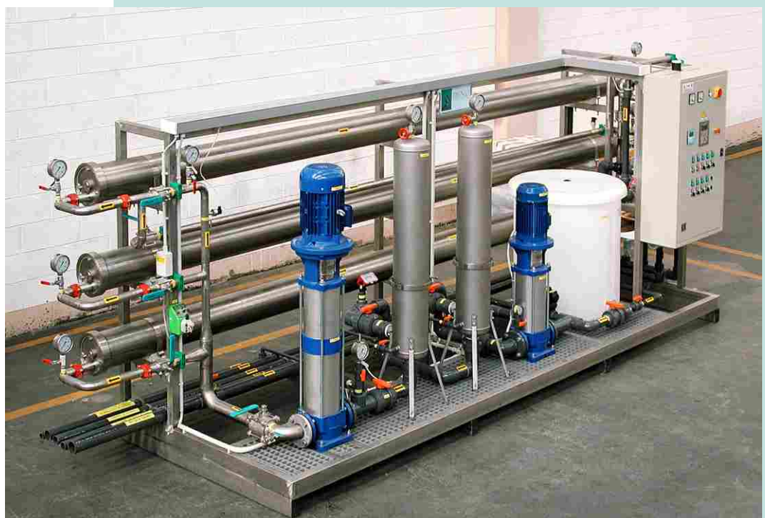
Reverse Osmosis unit - 15 mc/h
