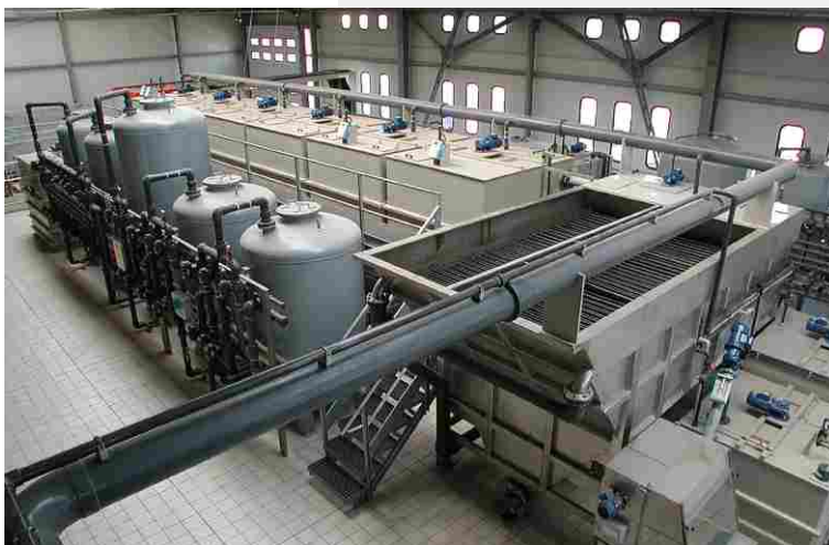
Wastewater treatment plant - 20 mc/h
