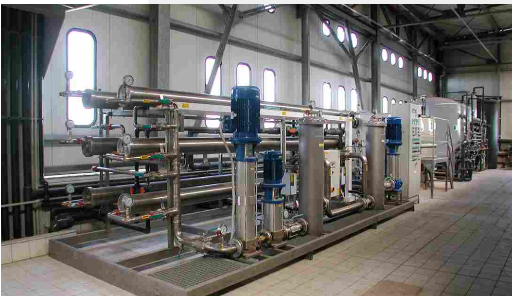
Reverse Osmosis section - 30 mc/h
